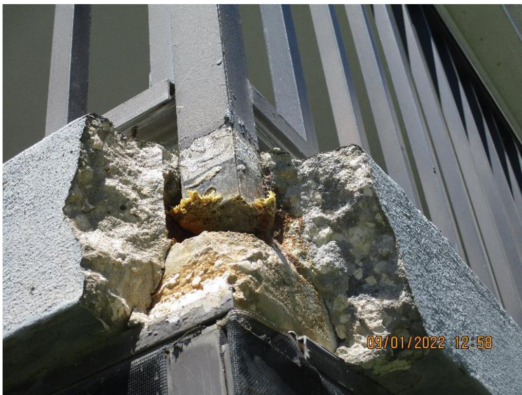
Concrete damage at foam-filled rail post
