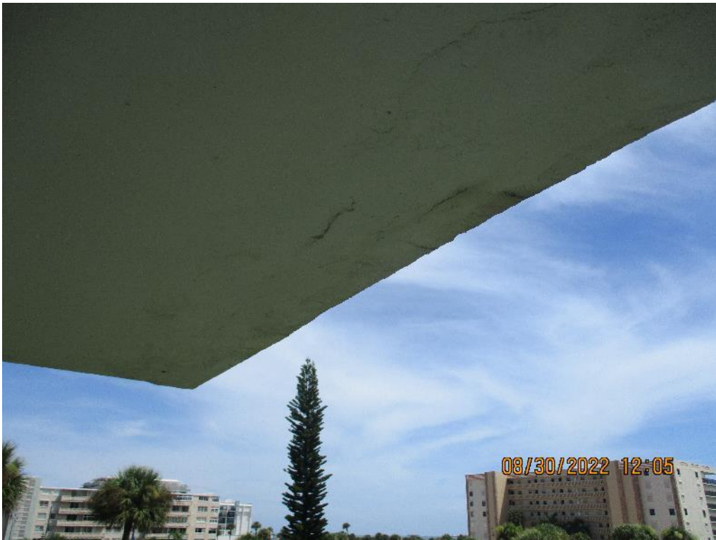
Edge spalls at the ceiling due to reinforcing steel corrosion
