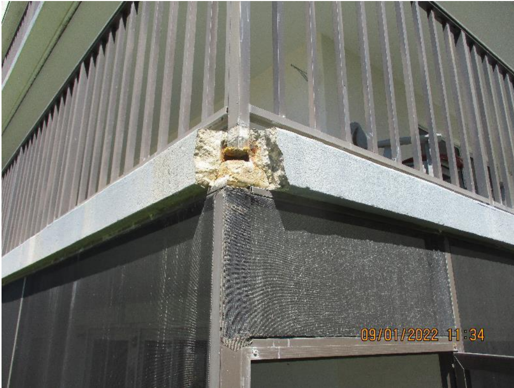
Cored railing causing edge spalling
