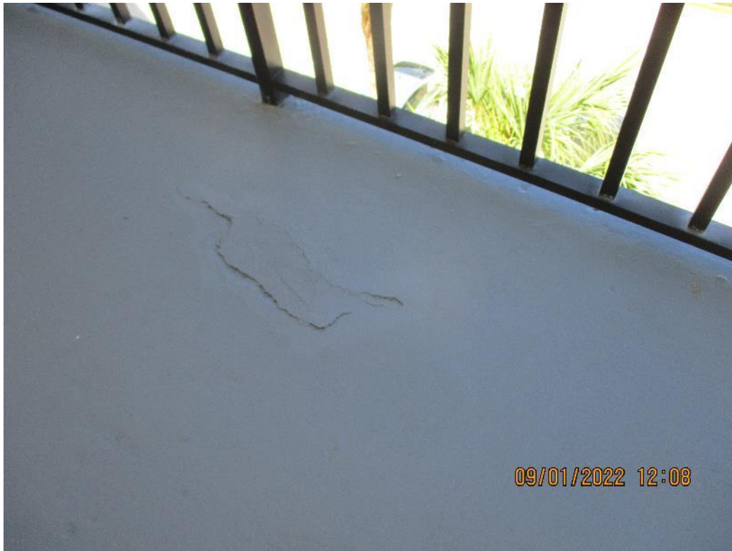
Surface spall along walkway
