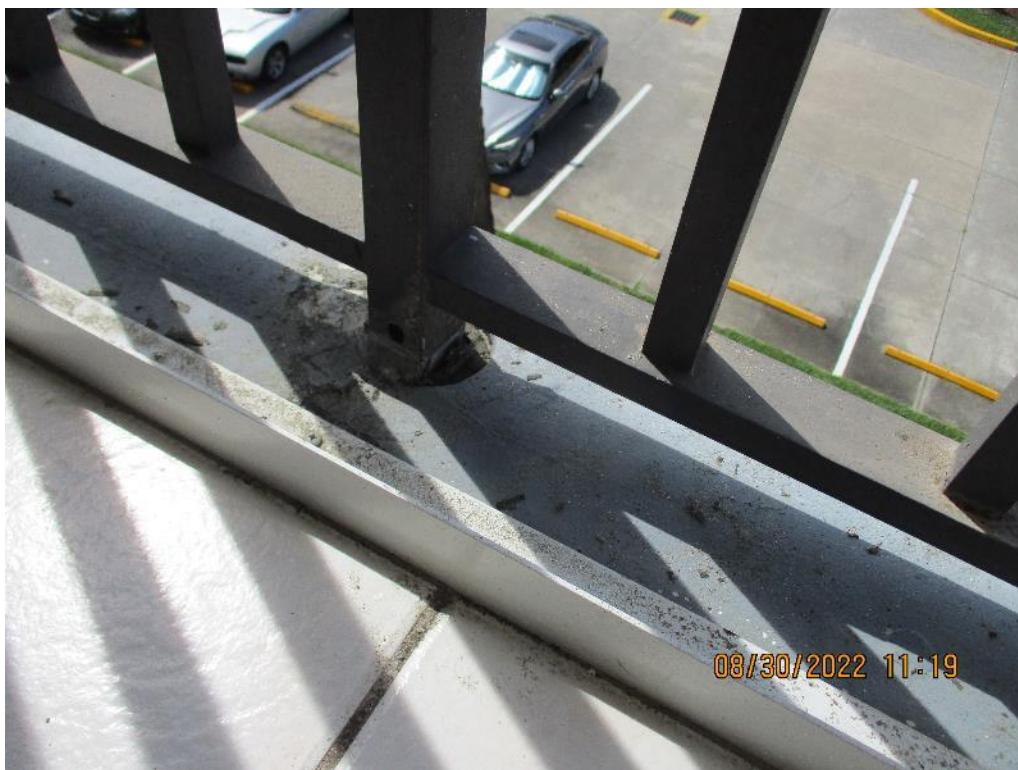
Railing core starting to fail
