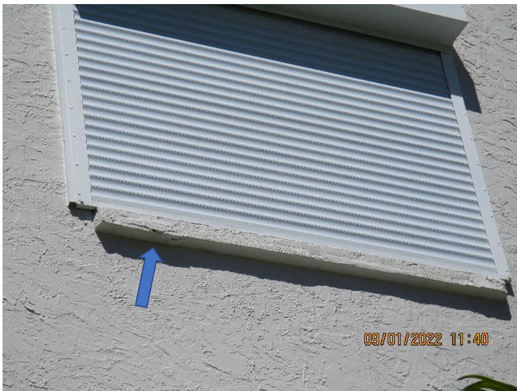
Window sill spall on building exterior
