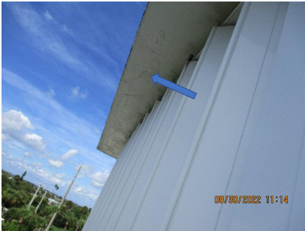
Balcony slab edge spall repair in failure
