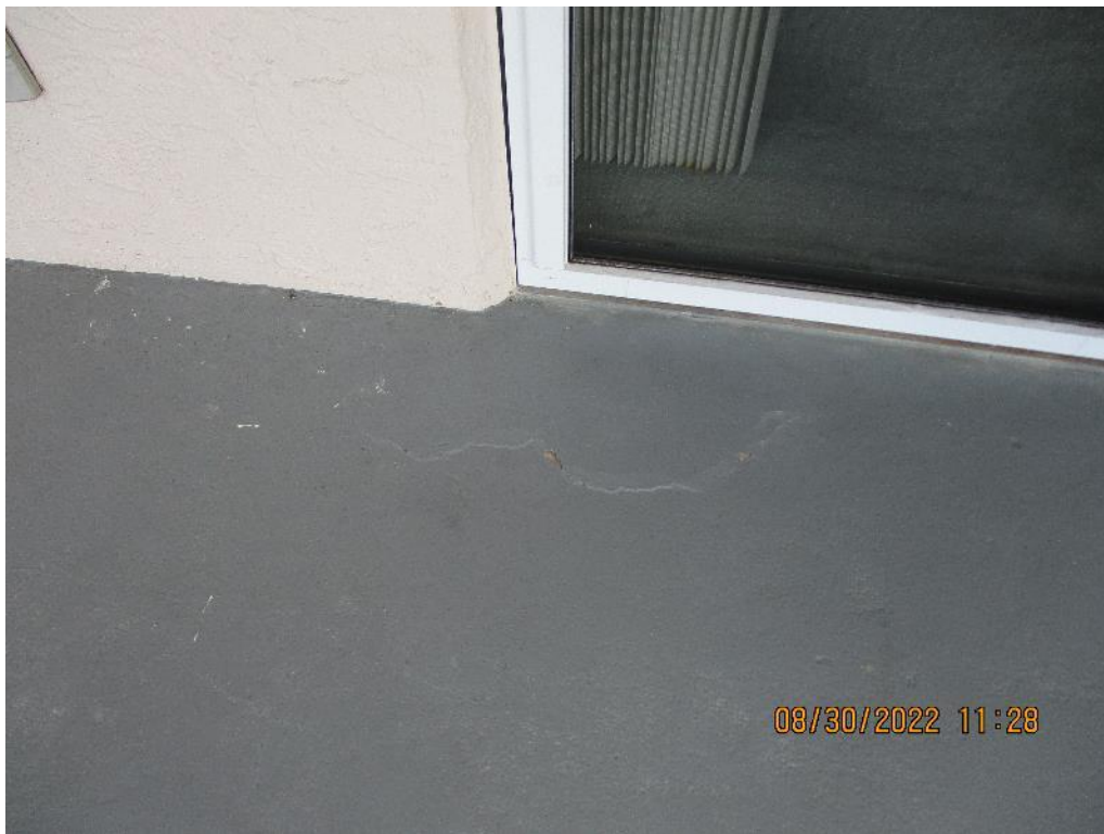
Concrete spalling at sliding glass door
