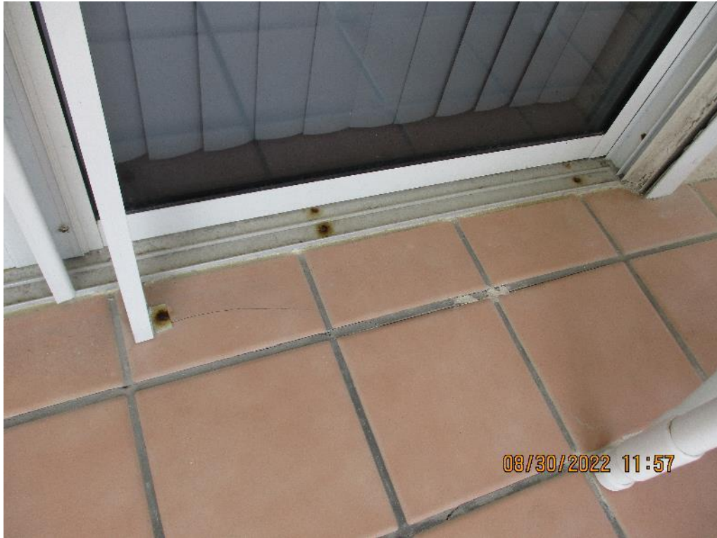
Corroded fasteners on sliding glass door and shutter tracks; cracking tile indicative of spalling below
