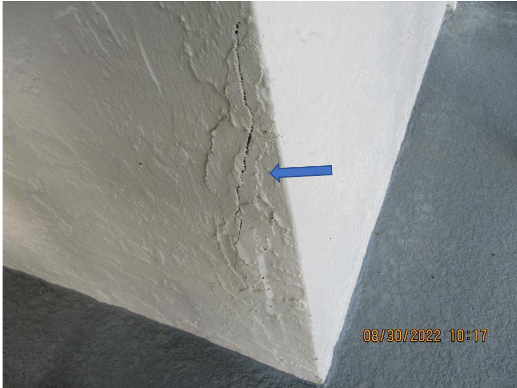
Column spall due to reinforcing steel corrosion (Unit 151)
