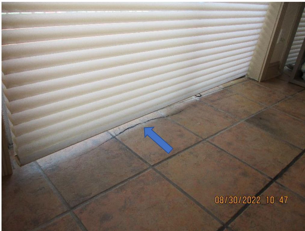
Interior tile cracking indicative of spalling below
