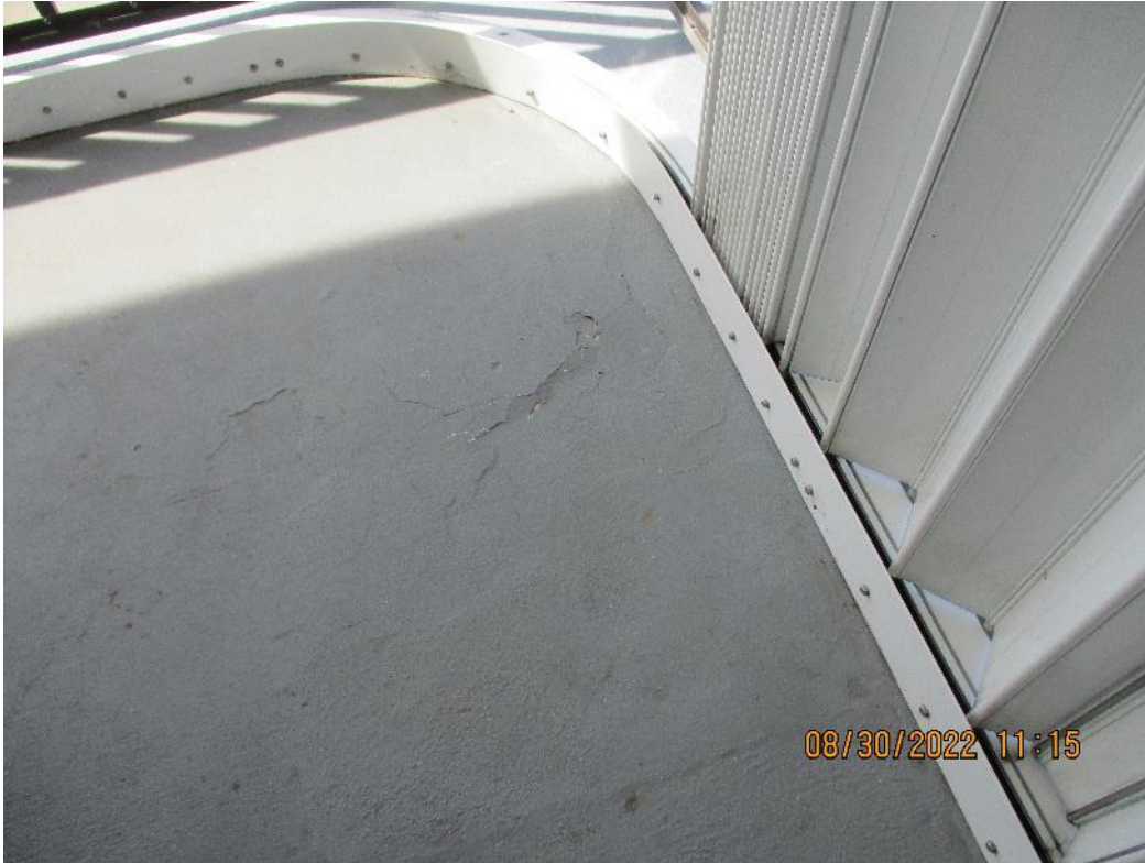
Floor surface concrete spalling due to reinforcing steel corrosion
