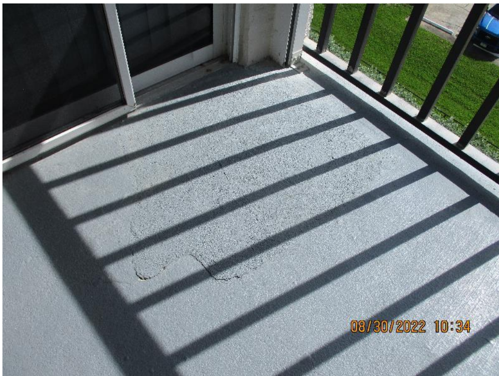
Past spall repair in failure
