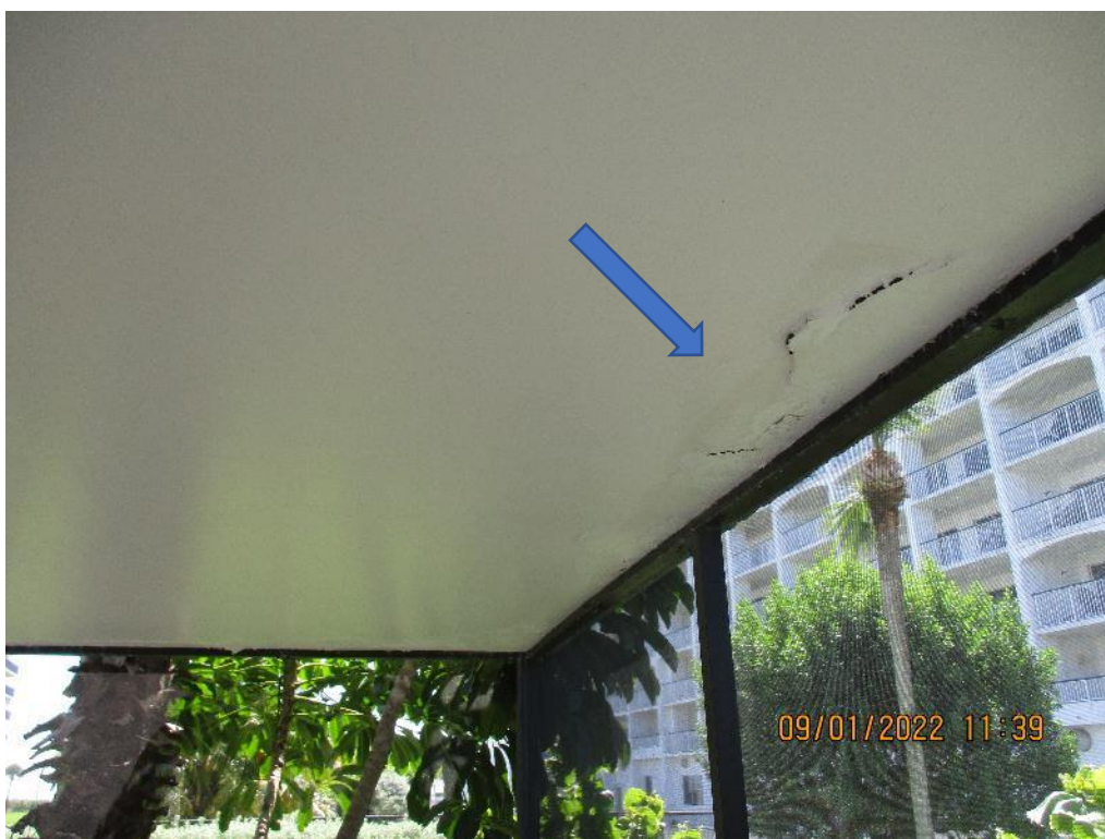
Concrete spalling due to reinforcing steel corrosion at balcony edge
