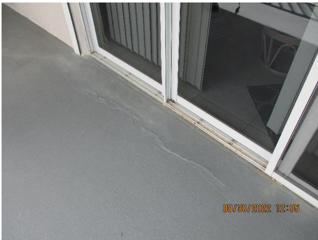
Concrete spalling at sliding glass door
