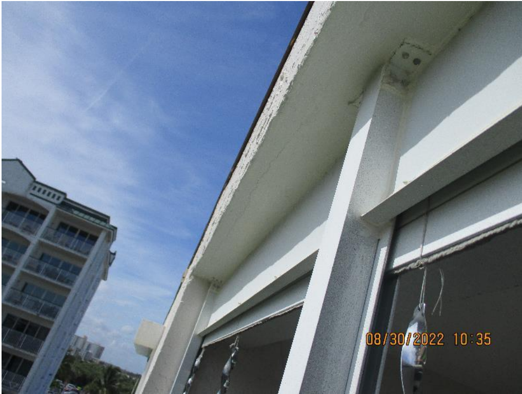
Edge spall along roof
