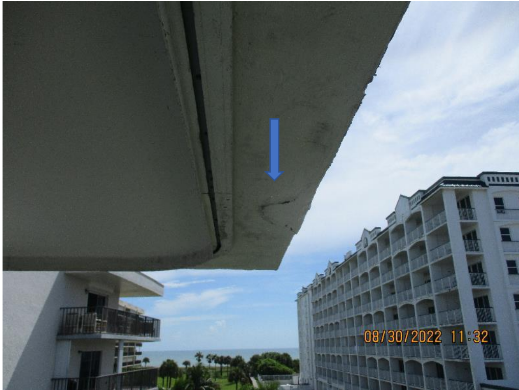
Edge spall on ceiling due to reinforcing steel corrosion
