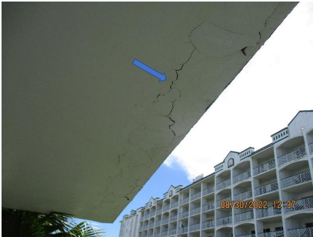
Concrete spalling along balcony edge due to reinforcing steel corrosion
