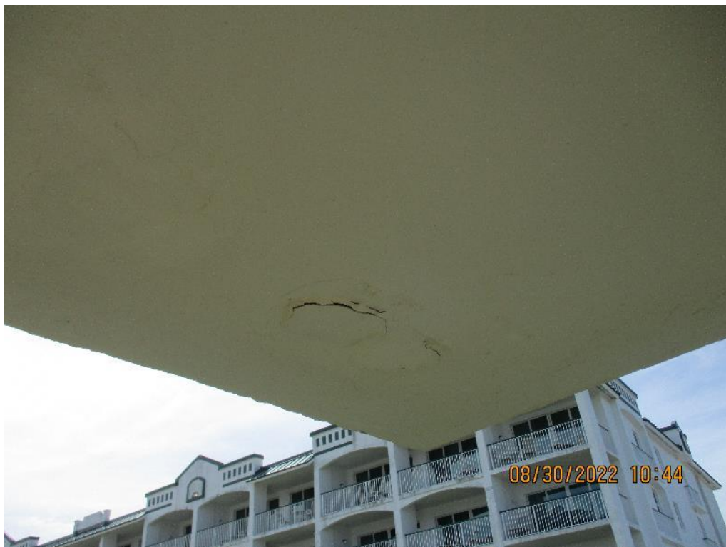
Example view of ceiling spall due to reinforcing steel corrosion
