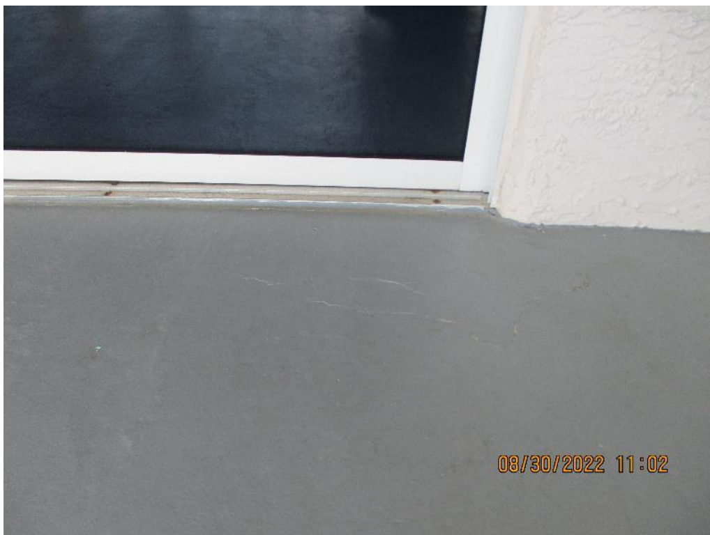
Concrete spalling at sliding glass door
