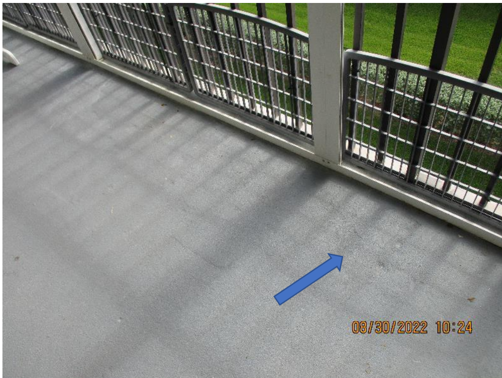
Floor spall due to reinforcing steel corrosion at blocked shutter drainage
