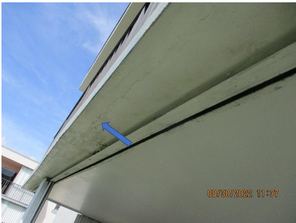
Edge concrete spalling due to reinforcing steel corrosion
