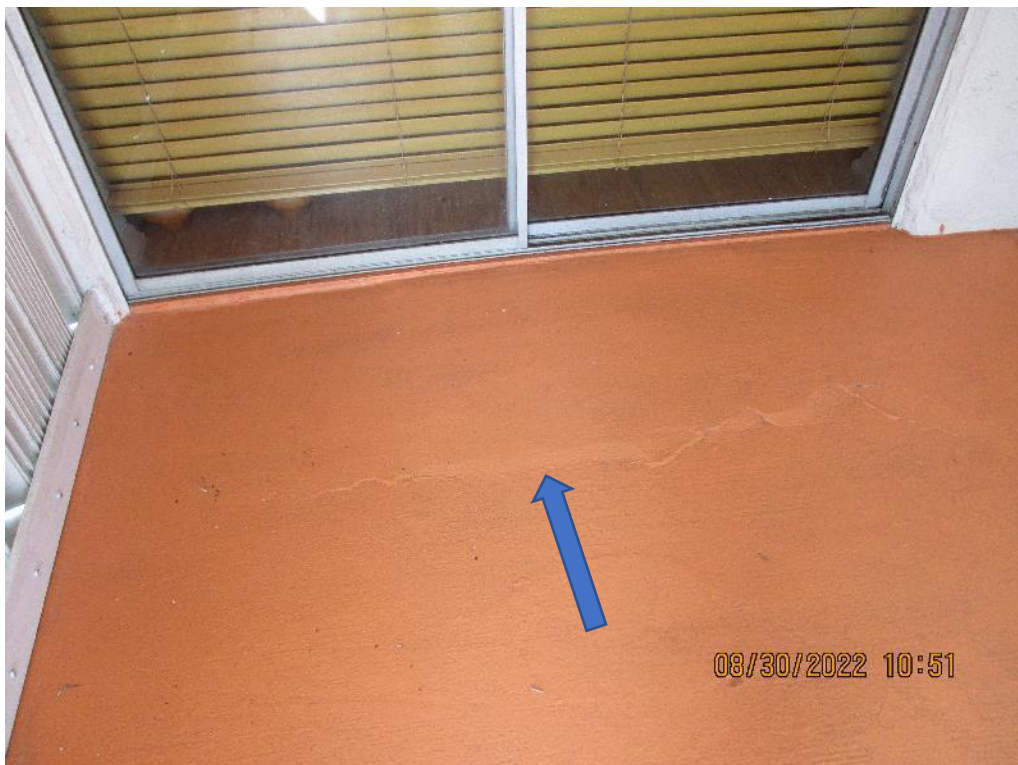
Example view of floor concrete spalling at sliding glass door due to reinforcing steel corrosion (Unit 203)
