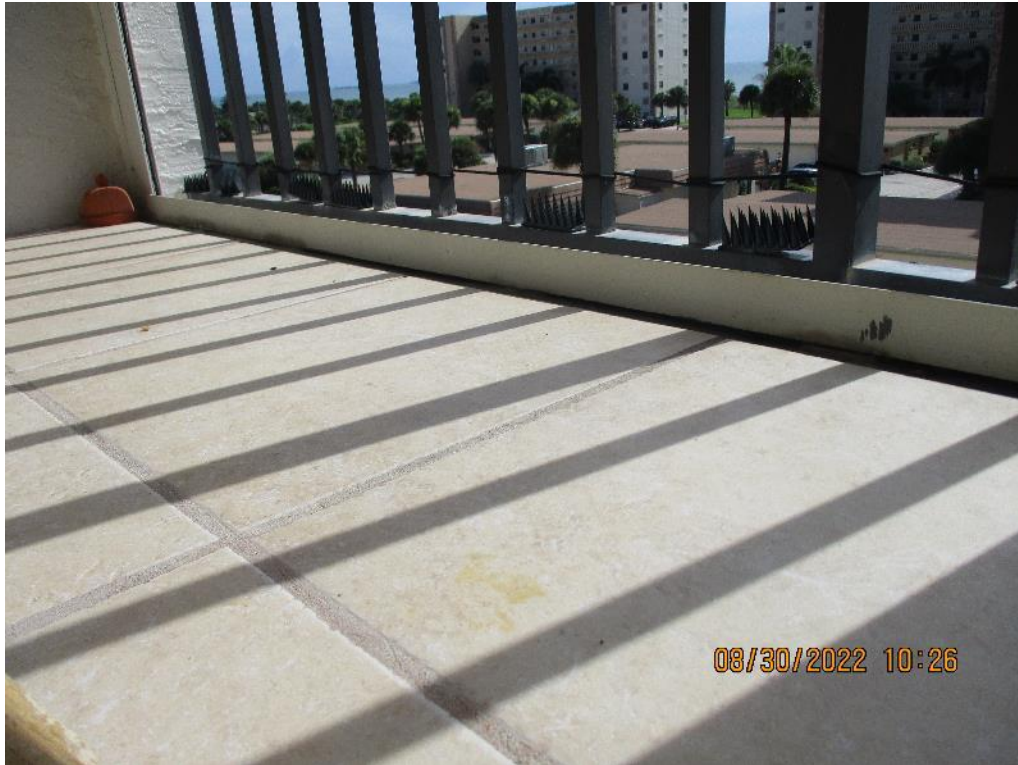
Drainage inhibited by tiles and hurricane shutters without any shims under tracks
