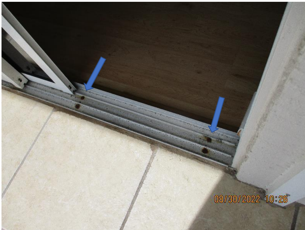
Corroded fasteners in sliding glass door track, allowing saltwater intrusion and structural damage
