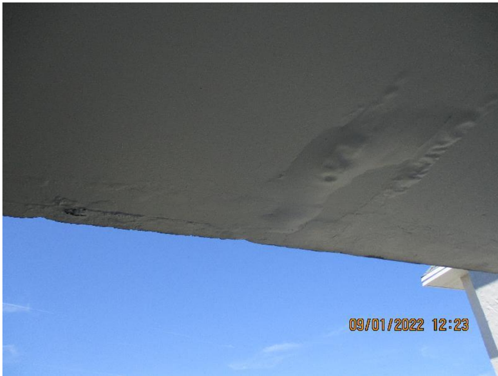
Example view of apparent water intrusion at walkway ceiling
